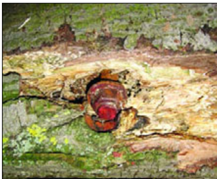
Decay around a through-bolt in lime (Tilia spp).
